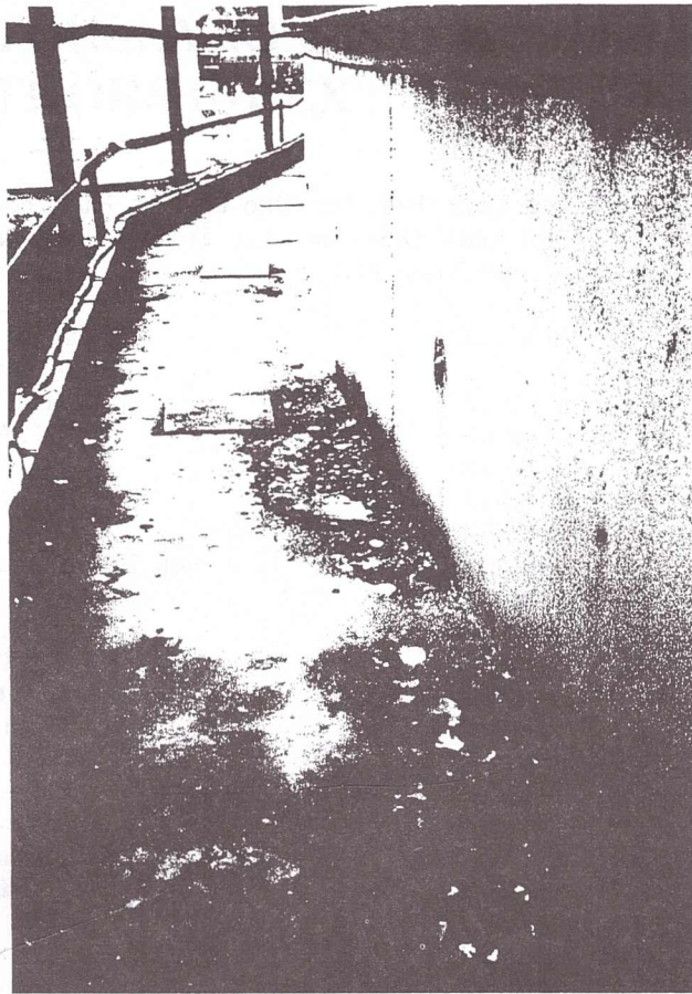
Fig. 4 Tank shell corrosion in the area near the plate wind girder
