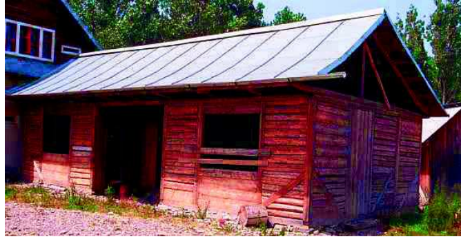
Fig. 8. Block Timber Infill Wall Sample
